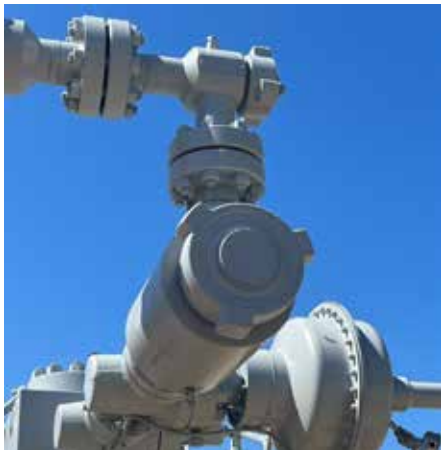
Hundreds of plug catchers have been installed in the field so far
